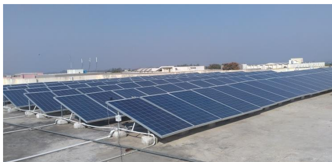
Figure1. Installed 100 kWp solar rooftop at the location
